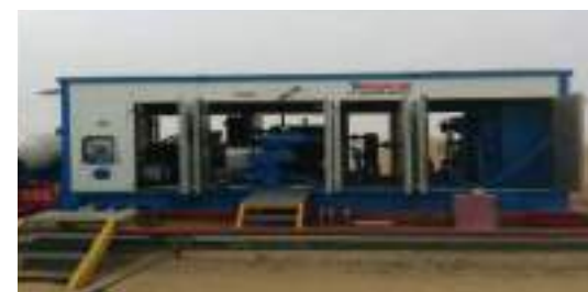
Sour Gas Compressor Unit
