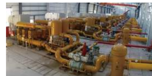
Natural Gas Gathering/Transferring
