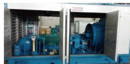
CNG Refueling Station
