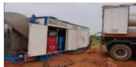
Flare Gas Recovery
