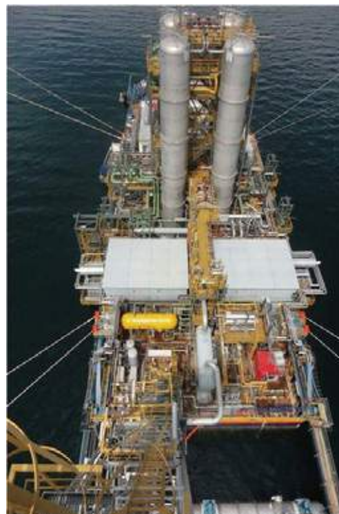
Two Compressor Packages on the Ship, Rwanda
